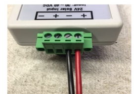
Solar Panel Input
